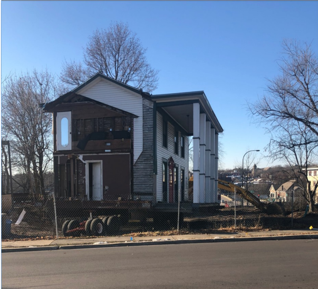
The Miller-Gully House west wing is ready to roll in December 2018. In the exposed wall note the horsehair plaster "keys" protruding between the lath and the typical haphazard placement of the "oversized" studs. The original clapboards are visible where a later chimney had been placed. The columned high roofed porch is an awkward 20 th century embellishment.
